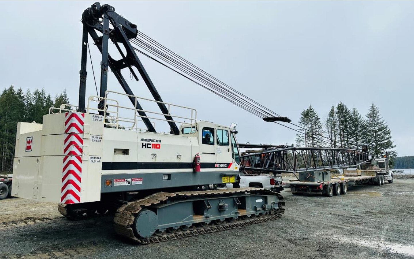
A large crane getting ready to drive in the piles beside the boat ramp.
