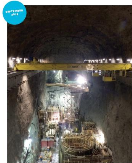
Powerhouse view from the service tunnel in September 2016. InPower BC, a subsidiary of SNC-Lavalin, consists of a team of contractors that includes Aecon Group (civil work), Frontier-Kemper (rock drilling and blasting), and General Electric (turbine/generator). With approximately 2.2 km of underground tunnels, and a powerhouse cavern that's 10 storeys high and as long as a football field, we removed about 300,000 cubic metres of rock. This picture shows the powerhouse cavern in September 2016.
