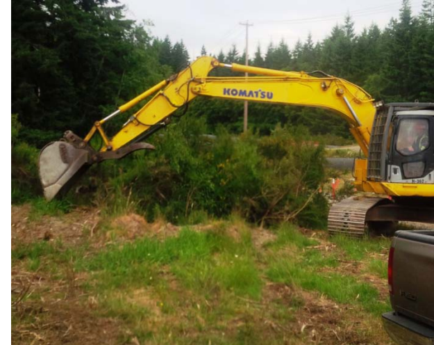
The first “ground breaking” on June 23 with brush removals for the preparatory works.
