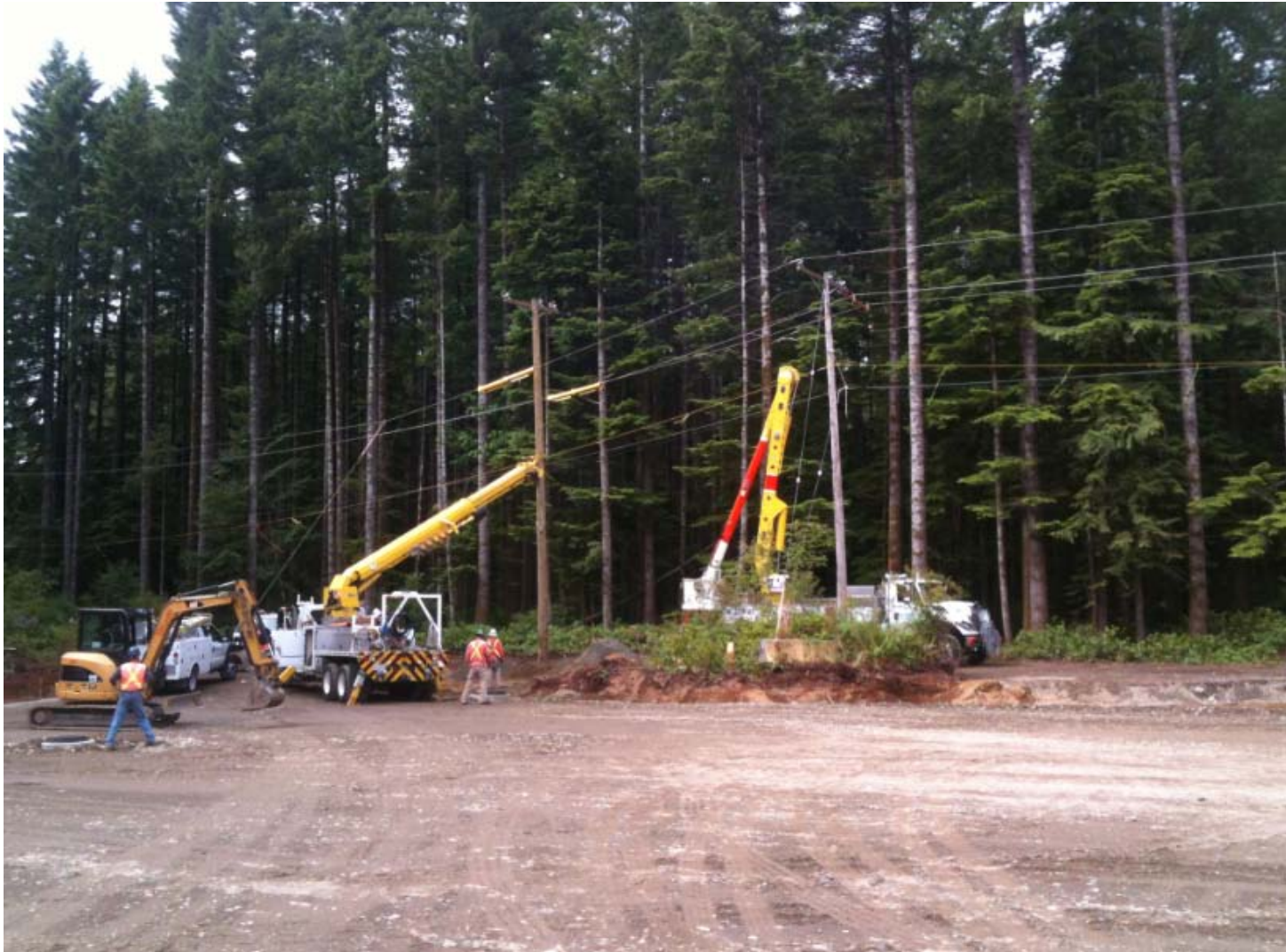
Moving a power pole where the new access road enters the parking lot.
