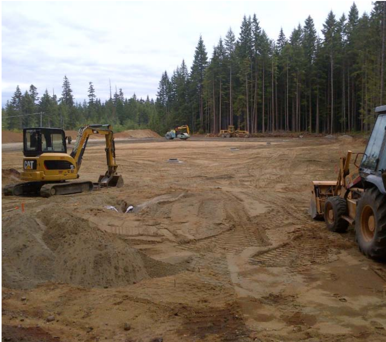
Completed drainage work (see manholes) and beginning of parking lot sub-base material.
